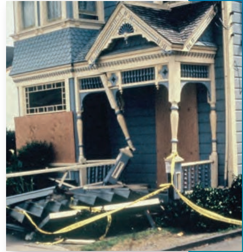
This older home collapsed after earthquake shaking damaged its crawl space (cripple) walls.
